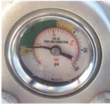
Example of Pressure Gauge damage
